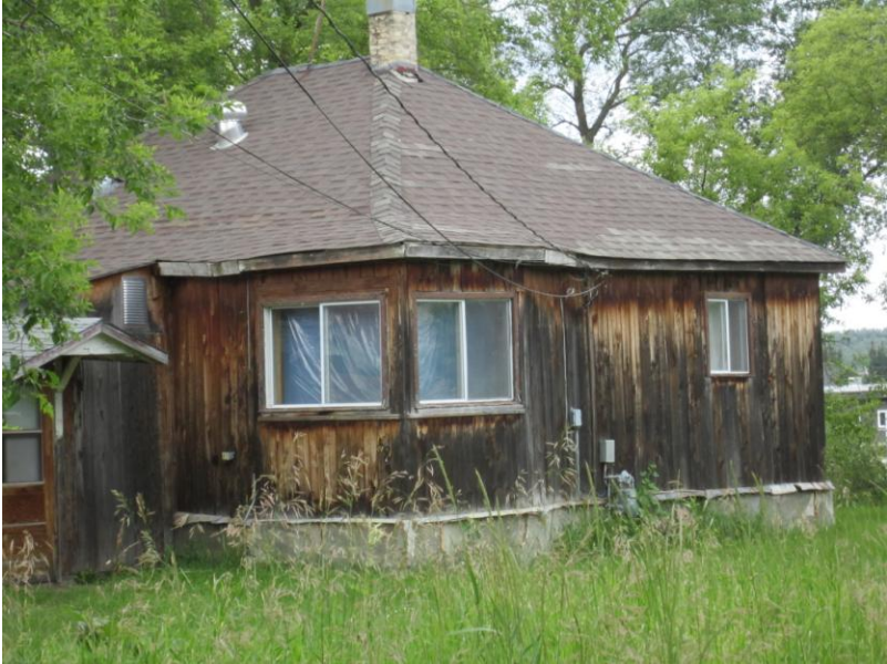
Figure 5: Derelict House in Minnedosa MB
